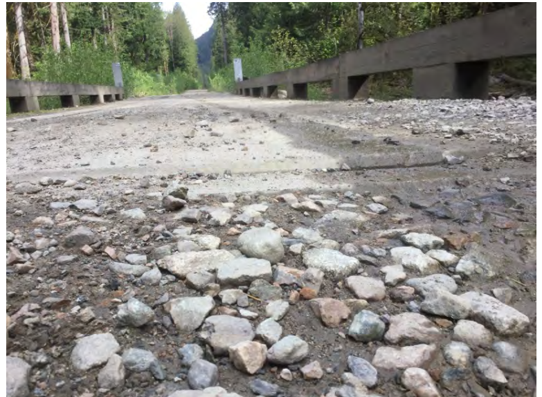
Left bank ballast wall installed 30mm lower than deck panels
