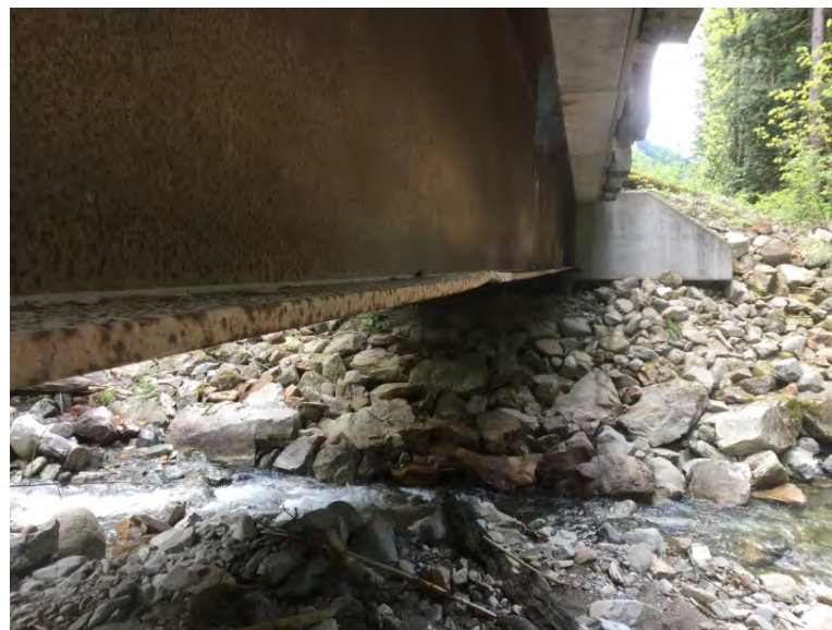
Some damage noted to bottom flange of downstream girder
