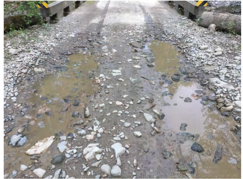
No surfacing at left approach
