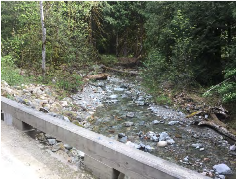
Upstream from Crossing, note debris in stream
