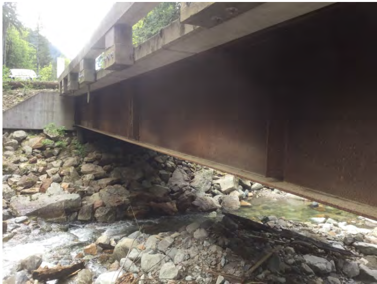
Stiffeners on outside of upstream girder but not downstream girder
